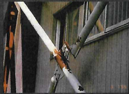
Rupture of diagonal brace joint
