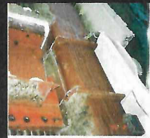
Rupture of welded beam-column joints
